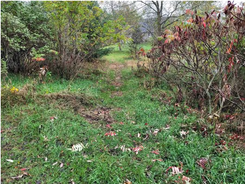
Photo #10 – Low area at right abutment, looking downstream
